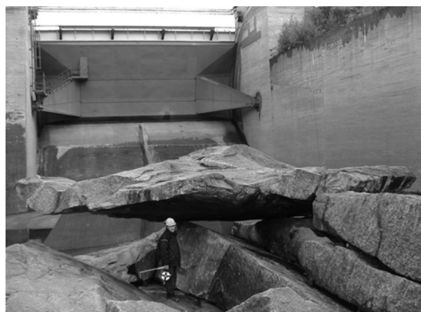
Figure 1. Eroded block in the spillway channel of the Harsprånget hydropower plant.
