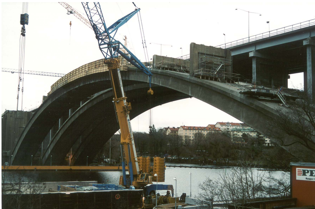
Figur 1.2 Bygget av det nya brospannet vid Traneberg i Stockholm (Foto: Jan Salomonson). Figure 1.2 Construction of the new span of the bridge at Traneberg (Photo: Jan Salomonsson).
