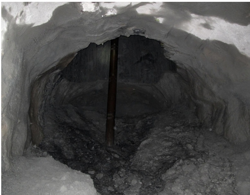
Figur 8. Kvarvarande borrsträng i personschaktet efter fallet. I bilden syns också hur borrkax tryckts ut i orten av fallet. The remaining drill rod standing on top of the rock plug in the personnel shaft. The picture also shows how drill cuttings have been pushed out in the drift caused by the fall of the reamer.
