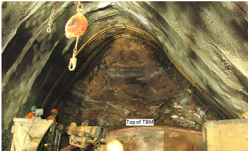
Figure 18: Overbreak from tunnel roof analyzed in Figure 17.
