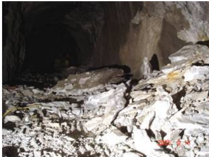
Fig.4 rockburst in access tunnel
