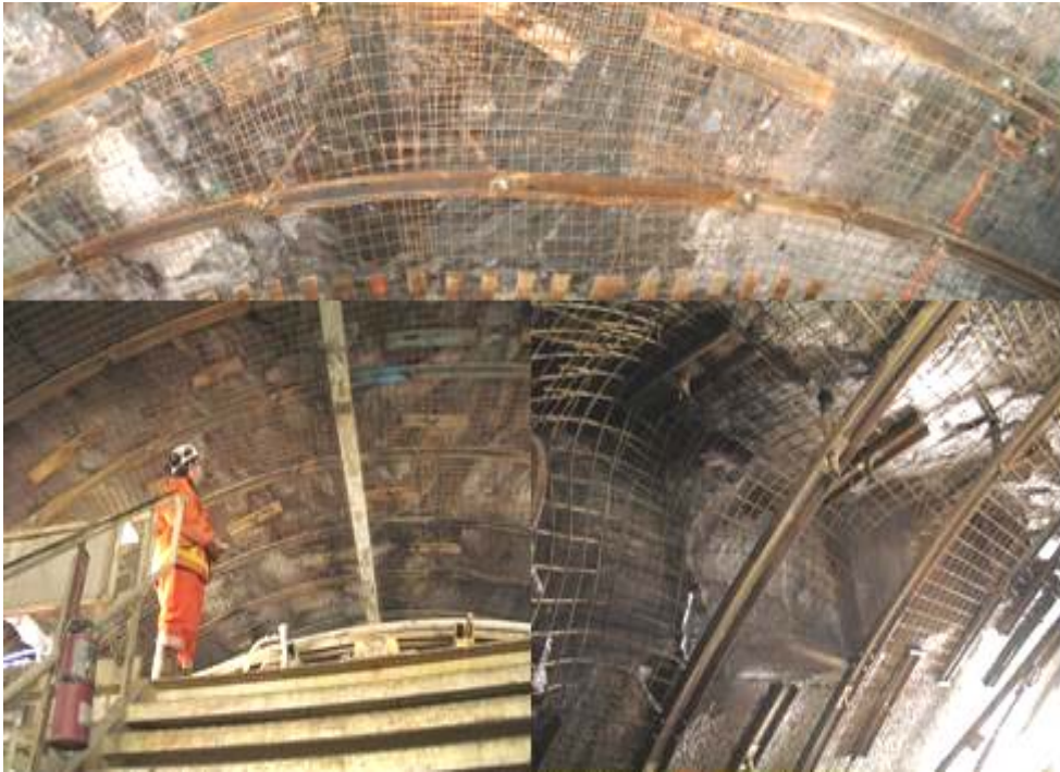
Figure 3: Overbreak as observed in the upper units in the Niagara Tunnel Project (Perras and Diederichs, 2009).
