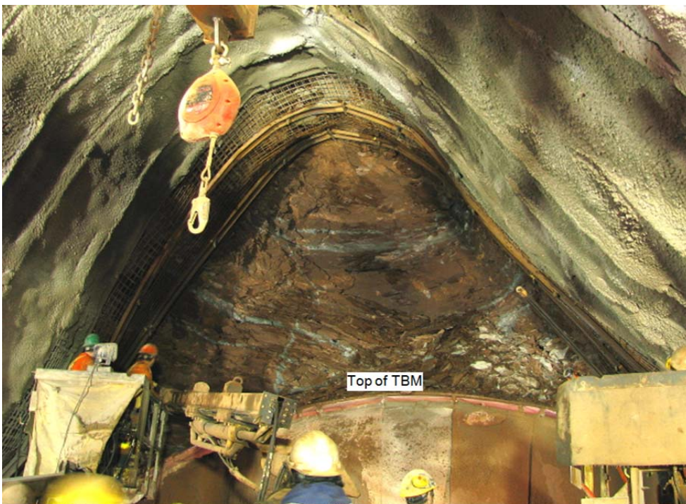
Figure 4: Overbreak as observed in the Queenston Shale on the Niagara Tunnel Project (Perras and Diederichs, 2009).
