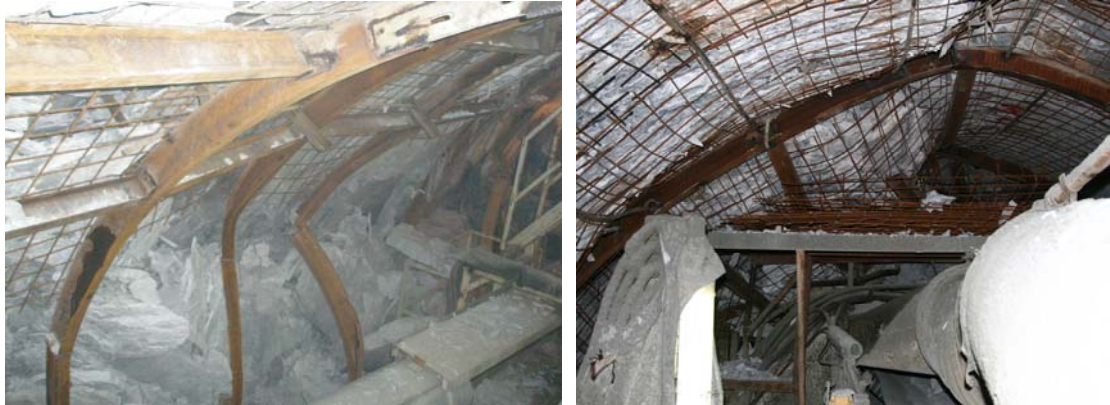
Fig.5 Rockburst in the drainage tunnel.
