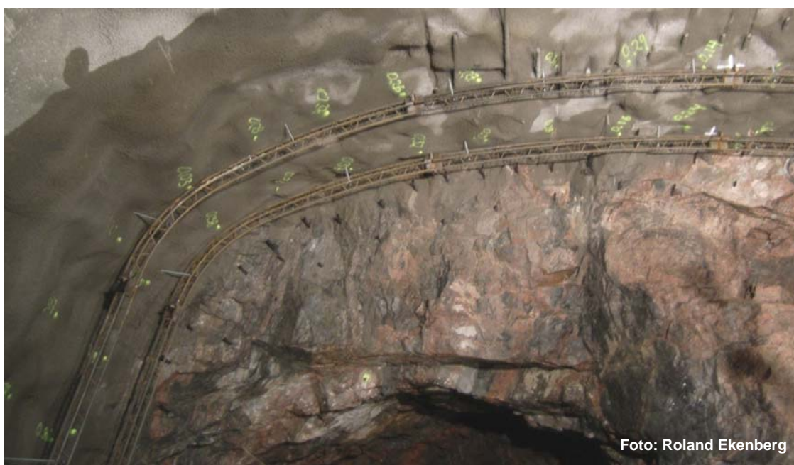
Figur 6. Injekteringsbara stag och gitterbågar, i nedre delen av fotot syns pilottunneln vidare Figure 6. Injection anchors and lattice girders, the pilot tunnel ahead is seen in the lower part of the photo
