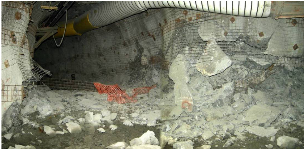
Figure 6 Breaching of the lower wall support could be observed frequently, irrespective of the wall support element combination, excavation geometry or accompanying structure. This demonstrates the need to consistently install burst support to the floor .
