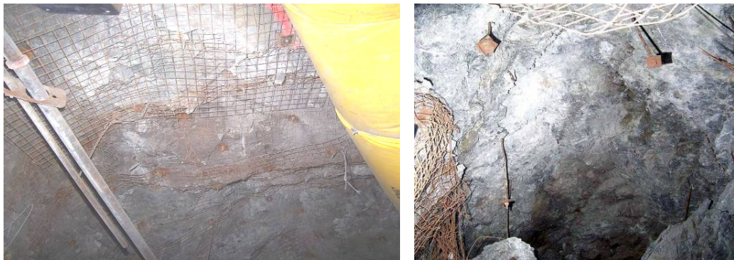
Figure 2 Left – Back of overcut 2 days before 1.8 Mn event showing Xstrata Nickel’s 2-tier rockburst support system, comprising 2.4m x 7/8-inch resin-grouted rebar and welded screen plus lines of heavy gauge screen strapping and resin-grouted cone bolts aligned across the drift and spaced every 1m or so; Right – domed back and South wall of burst site with remnants of sheared-off bolts and some intact ones with plates sheared through the screen; most of the installed support was buried by the groundfall.
