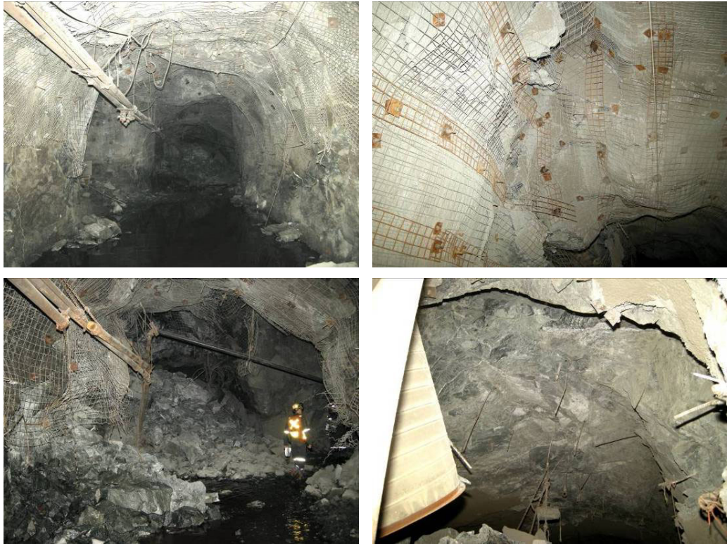
Figure 4 Comparison of ground support systems in use: Bolts & Screen vs 75mm FRS + Rebar & Screen+Screen Straps & Modified Cone Bolts; Top – as installed; Bottom – local damage sustained by rockburst.
