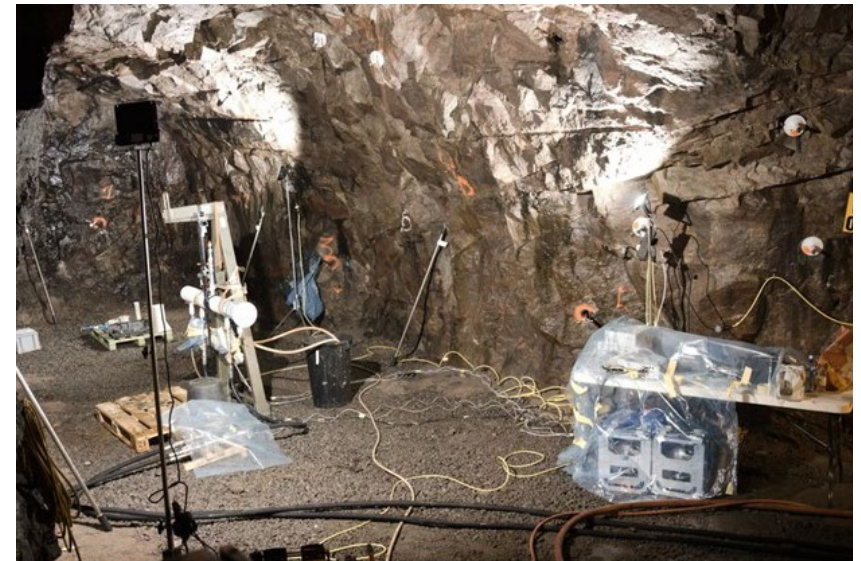
Distribution unit at Äspö HRL
