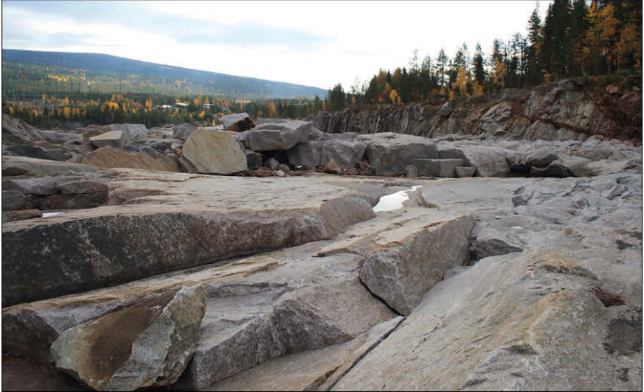
Figure 11. Dam 1 spillway block erosion.
