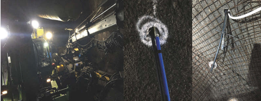
Figure 10: Installation of extensometers. Hydraulic lift and cable bolter in the drift (left); toe with spring anchor (center), installed extensometer with packer waiting for grout (right).
