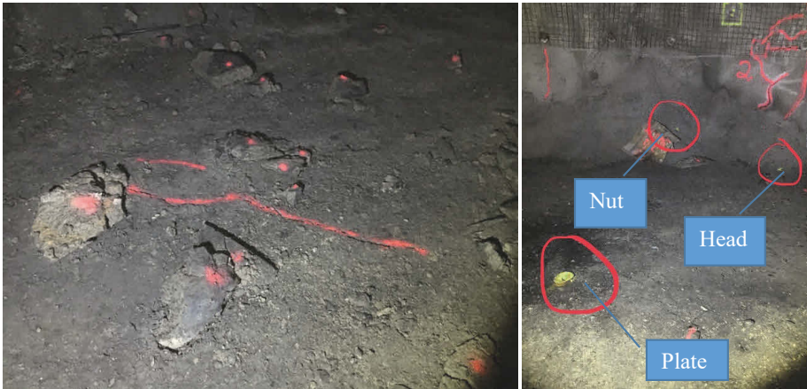
Figure 31: Fallen material painted on the floor identifies it as pre-existing (left). Bolt plate, bolt head, and nut painted as pre-existing (circled on right).
