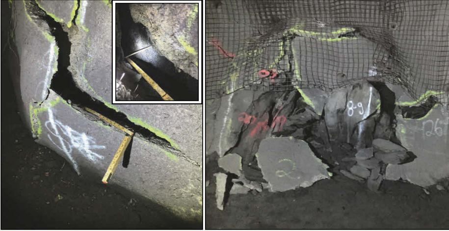
Figure 174: Buckling in the lower wall often caused wall damage and decoupling of the shotcrete from the rock.
