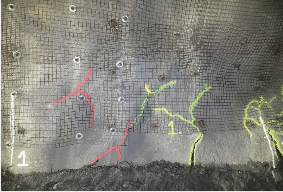
Figure 30: Example damage mapping section, crosscut 2800, Lw, Section 1, from 2019.05.23. White vertical lines and the white “1” are the section markers, yellow “1.” is a crack number. Colored crack painting occurred at different times to help show change between mapping periods.
