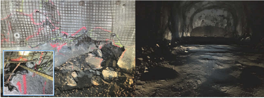
Figure 56: Excessive Lw deformation in 4090 S5 (left), large floor heave in S8 (right).
