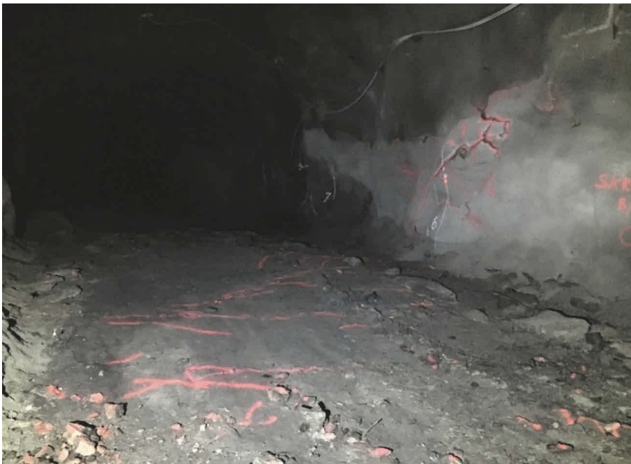
Figure 34: Crack propagation angling across the floor into the right wall of entry 4080.
