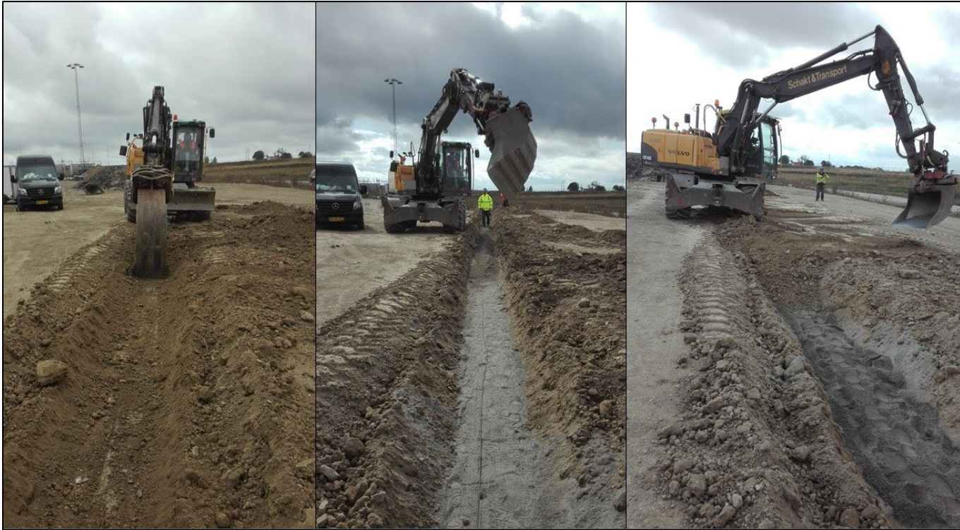
Pictures of the installation of the fibre optic cable in the ground: left, digging of the trench; middle, cable on top of sand layer; right, backfilling of the ditch with sand and excavated material.
