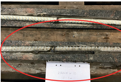
Figure 3-15. Core from bolt TASJ10 – the unfilled pocket, 30 mm deep and 400 mm long at the bolt length 0.4–0.8 m.
