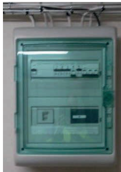
Figure 19. Power distribution board
