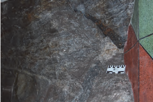
Figure 26. An example of a rock wall from Kungsträdgården platform where the fault surfaces were exposed (site Kungsträdgården (09) surface no. 005) indicated as 09-005 in Table 1.
