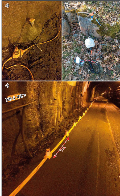
Figure 4. Examples of planted geophones in drill holes in the rock (a) in the tunnel and (b) on the surface. (c) The seismic landstreamer used in the tunnel in the downdip direction (known from drilling) of the NE-1-III fracture zone.
