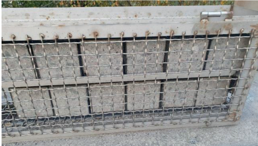
FIGURE A6.6. October 2021. Original cage. No damage to the concrete surface observable.
