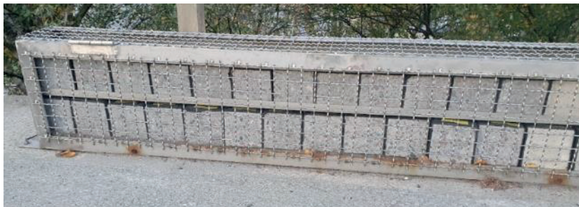
FIGURE A6.7. October 2021. Long cage all recipes, no obvious damage to the concrete surfaces. Rust starting to form on some of the threaded parts of the cage.
