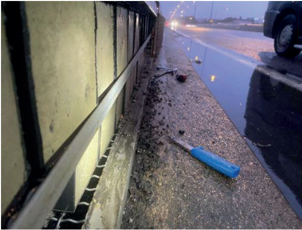
FIGURE 3.8. View looking back to Älvsjö, double lane going in both directions with a concrete barrier separating the traffic flow. Water and debris accumulate in this vicinity.
