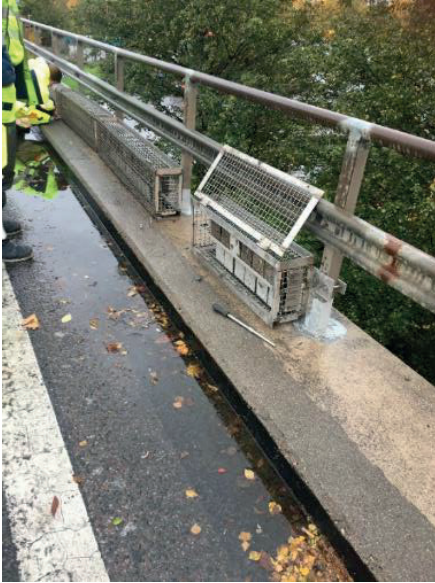
FIGURE 3.7. Autumn check of the specimens, the area between the raised edge beam and asphalt is rarely dry.
