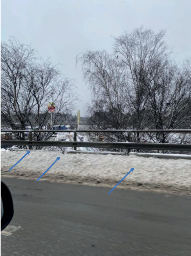
FIGURE 3.9. Driving past the field station 8th January 2022. Snow has accumulated on level with the top of the safety cages, see the blue arrows. The lane between the car and the edge beam, i.e. where the specimens are fixed, is a merging lane see [74].
