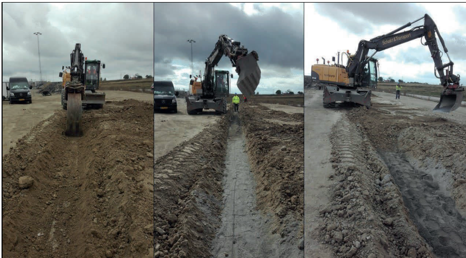
Figure 8 Pictures of the installation of the fibre optic cable in the ground: left, digging of the trench; middle, cable on top of sand layer; right, backfilling of the ditch with sand and excavated material.
