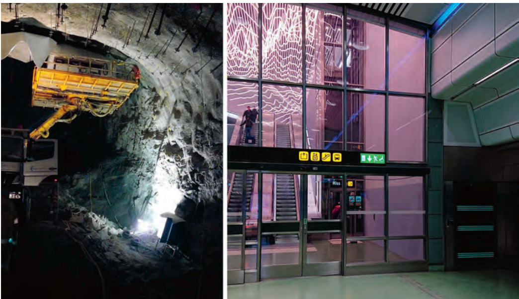
Fig. 1 Escalator shaft at the Odenplan commuter train station in Stockholm, Sweden. Temporary design situation during construction of the shaft (left) and permanent design situation when the station is in use (right)
