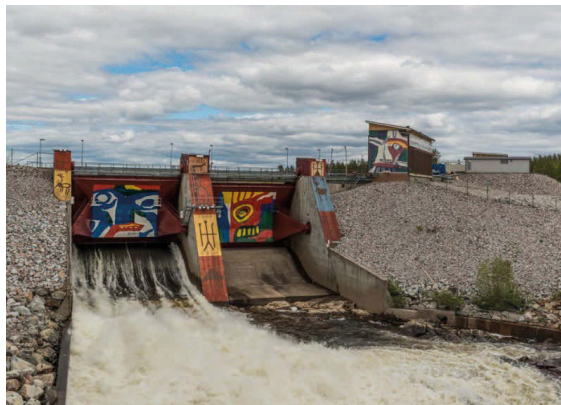
Figure 2.2. The spillways of Akkats in Lule älv River in northern Sweden are examples of concrete dam structures. (Photo: © Daniel Vorndran, 2015)
