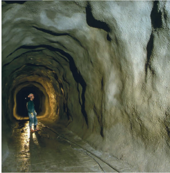
Figure 2.1. Tunnel lining of steel fibre reinforced shotcrete. Picture by courtesy of BESAB, Gothenburg, Sweden.
