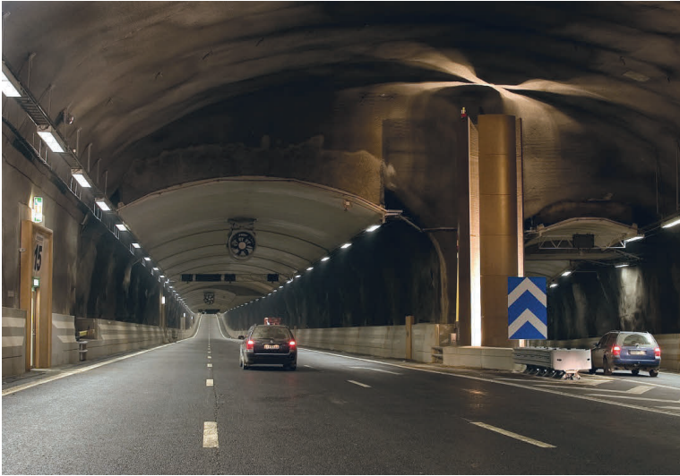
Figure 2.8. The Southern Link road tunnels, constructed with shotcreted drains. Photo provided by the Swedish Road Administration.
