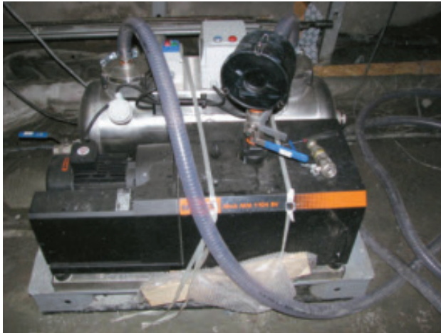
Figure 3-4. Vacuum pump from a sealing project in the Telia tunnels.
